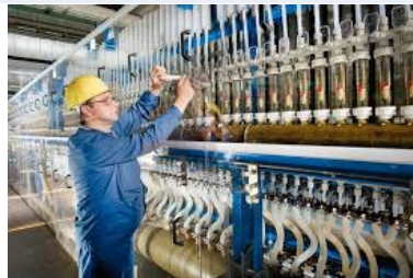
Electrolysis cell hall
